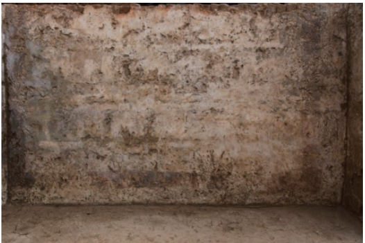
图一〇 东耳室南墙壁画颜料脱落
